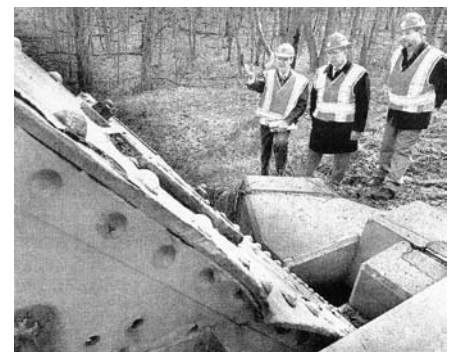
Rep. John Hall, center, DOT's Dave Bennett, left, and Deerpark Supervisor Gary Flieger examine the Cuddebackville Route 209 bridge, March 21, 2008
