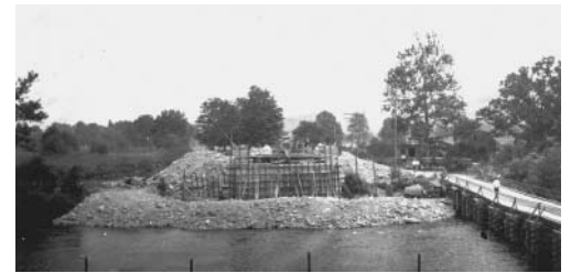
Construction of current bridge A temporary structure was built to facilitate crossing the river.
