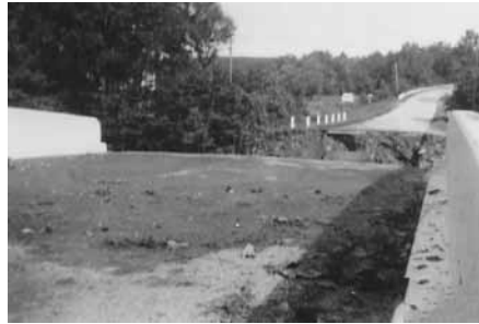
Route 42 washed out during the 1955 flood
